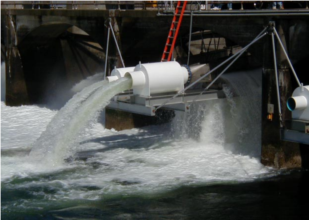
View looking northeast at the newly installed smolt chutes at the Ballard Locks. Equipped with electronic counters, these chutes provide the best route to the sea and should lead to improved survivability for smolts. --Photo by Fred Zingleman
